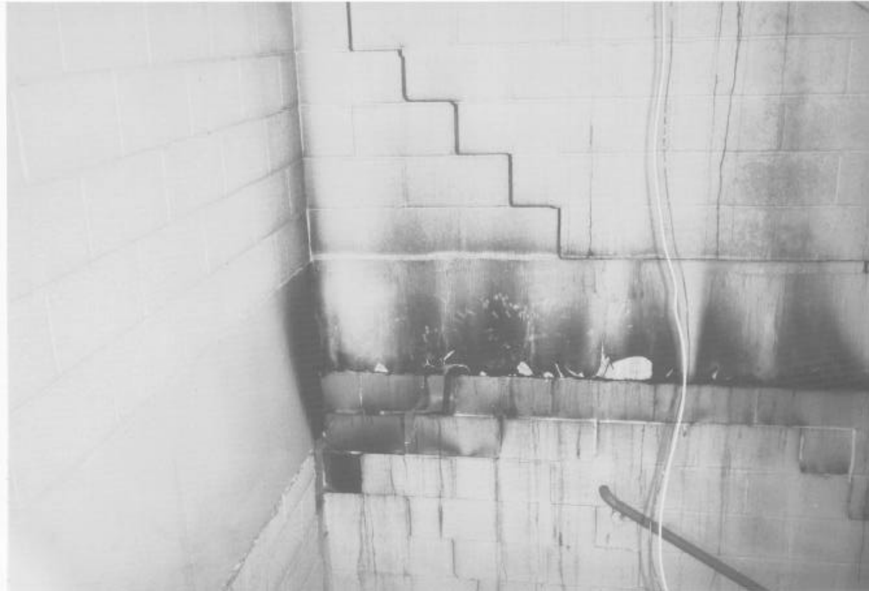
Fire tower between 25th and 26th floors. Note heavy fire and smoke damage.
