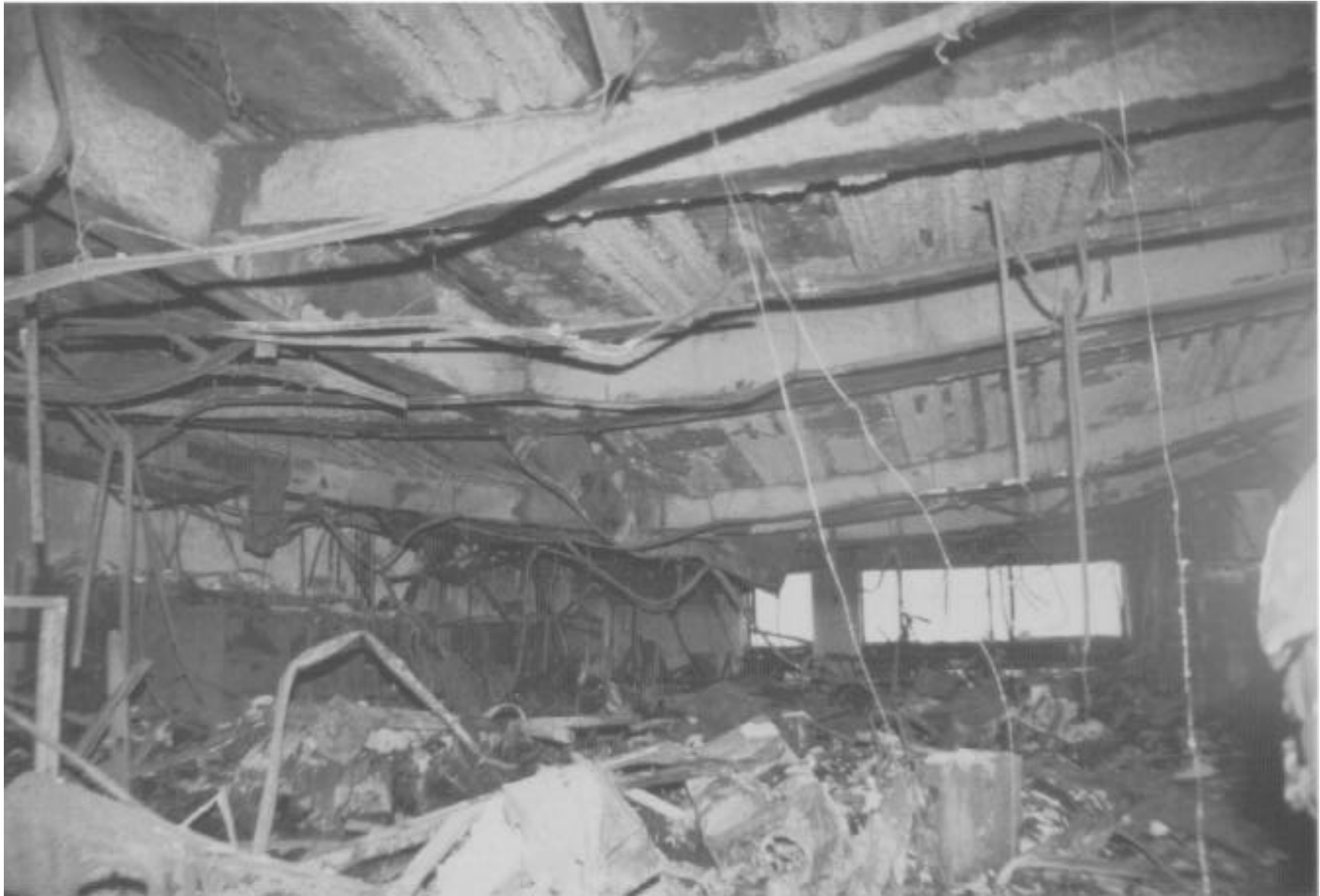
Here and in the next three photos are interior views of floor areas after the fire. Note the total consumption of the available fuel and sagging of the floor deck of up to three feet between columns.
