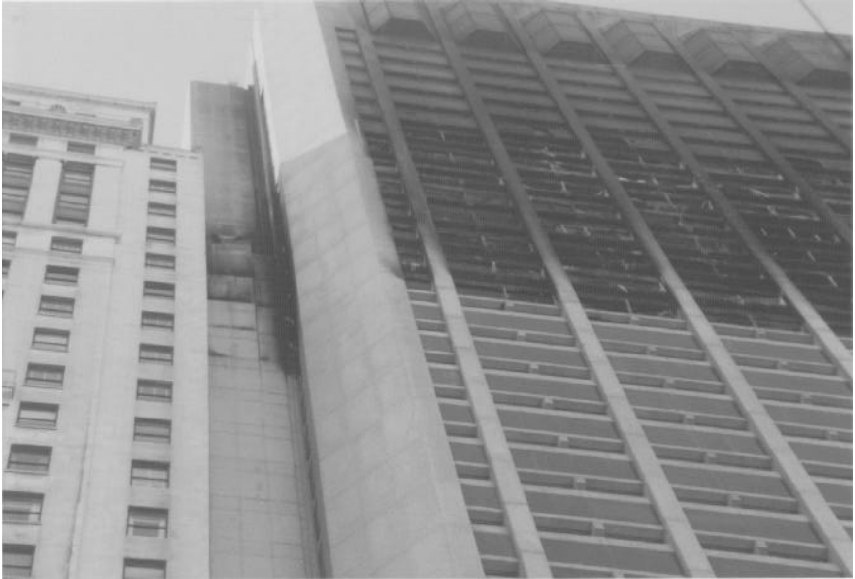
This stairway connected the One Meridian Plaza Building with the adjacent office building.
