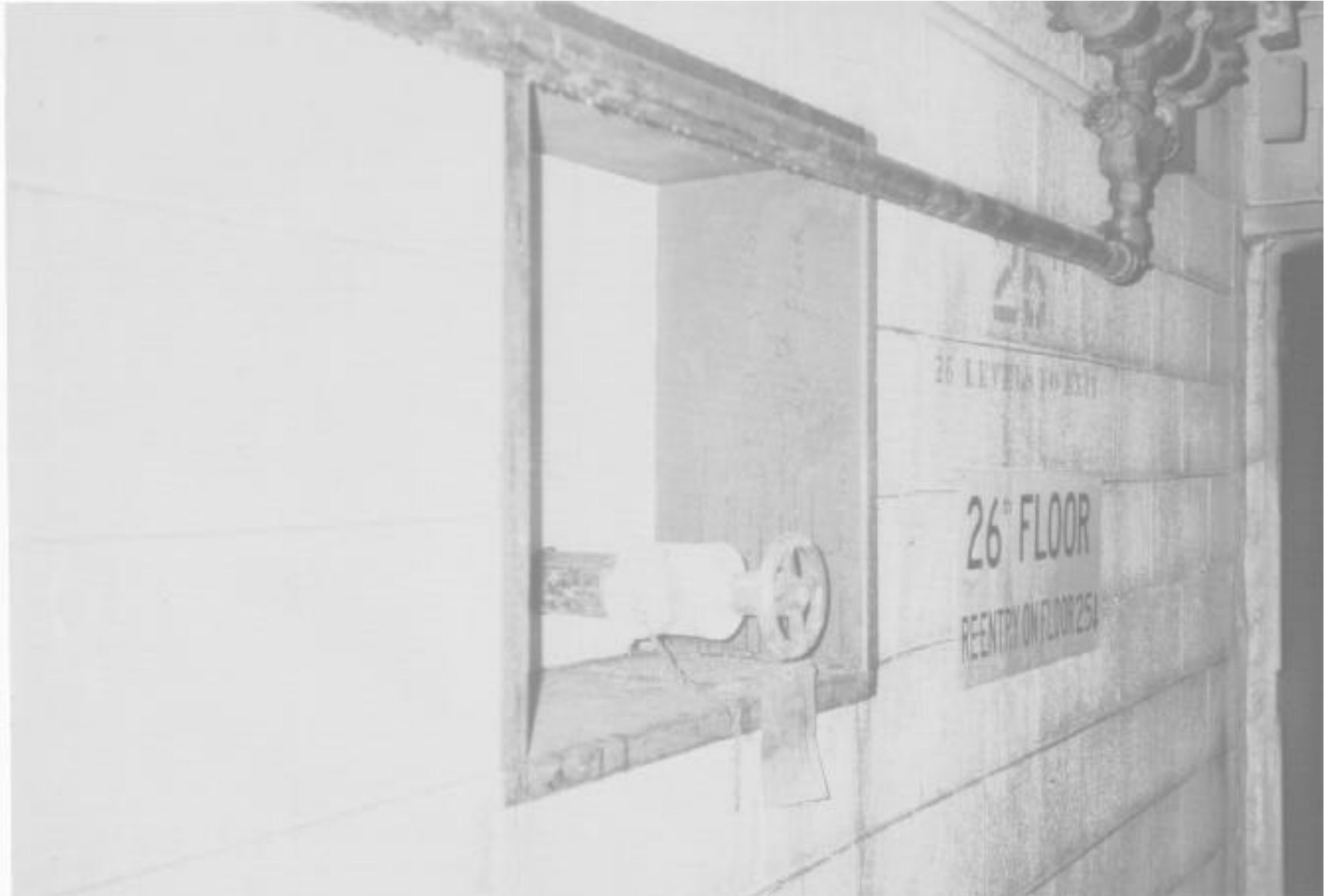
Standpipe hose outlet with pressure reducing valve (PRV), 26th floor.
